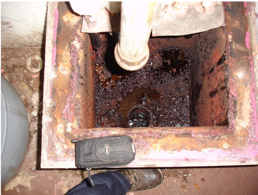
Fuel oil #6 entered corroded heating coils and flowed with condensate to floor drain that leads to sanitary sewer.
