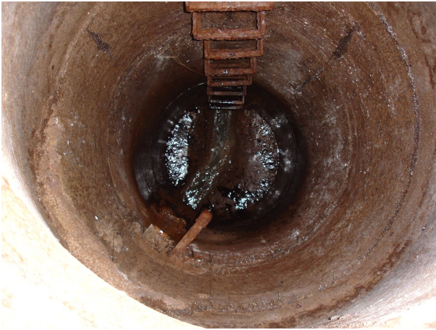
Typical view of a sanitary sewer manhole showing fuel oil at depth
