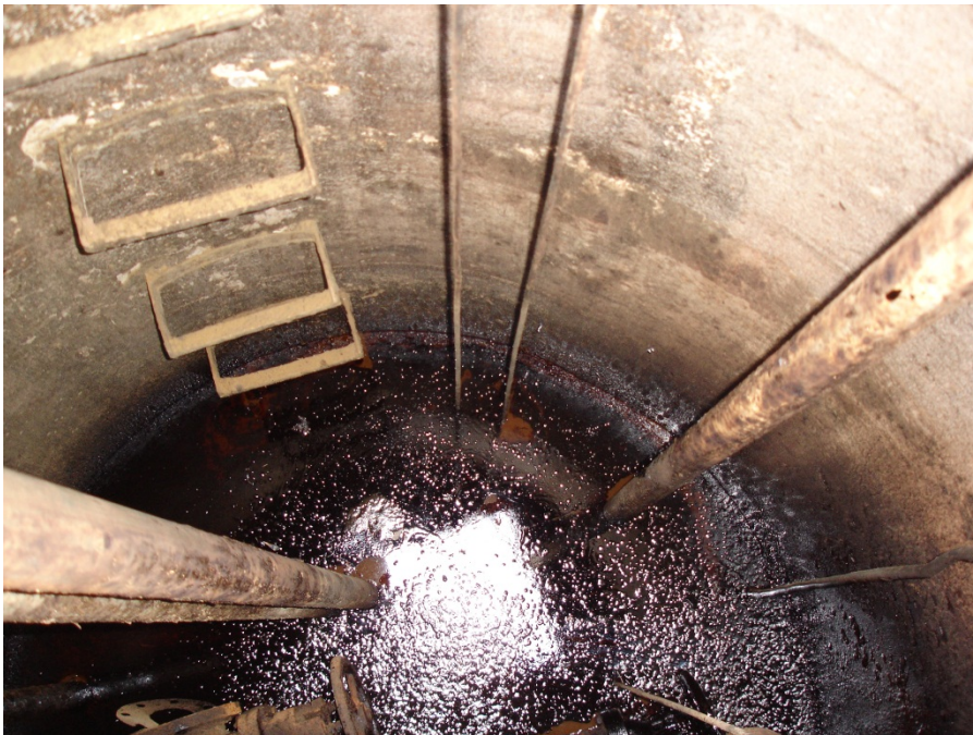
river side of the power plant at ~920' east up a hill to the sanitary sewer at ~955'.
