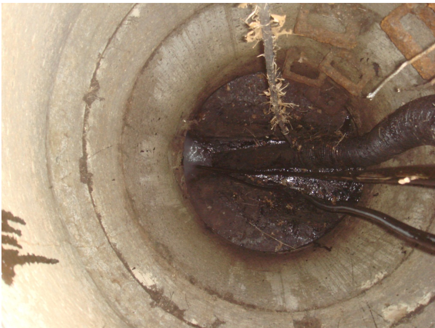
Vacuum hoses and jetter lines used to clean and recover fuel oil from the sanitary sewer
