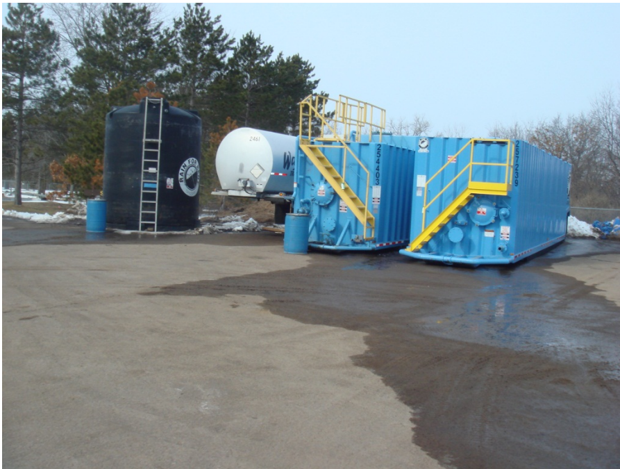
Contaminated water without a sheen was stored on site and disposed of under a Met Council discharge permit
