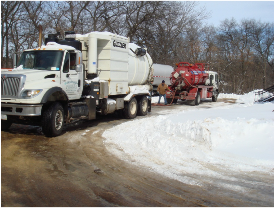
Contaminated water with a petroleum sheen was disposed of at Determan Fluid Solutions
