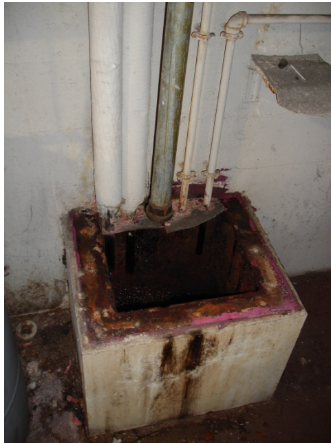
Piping at top of picture carries heating coil condensate water to floor drain at the power plant. The heating coils are necessary to make the fuel oil #6 flow.
