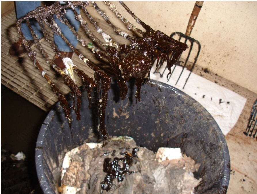
Fuel oil no. 6 "sludge" at WWTP pretreatment building
