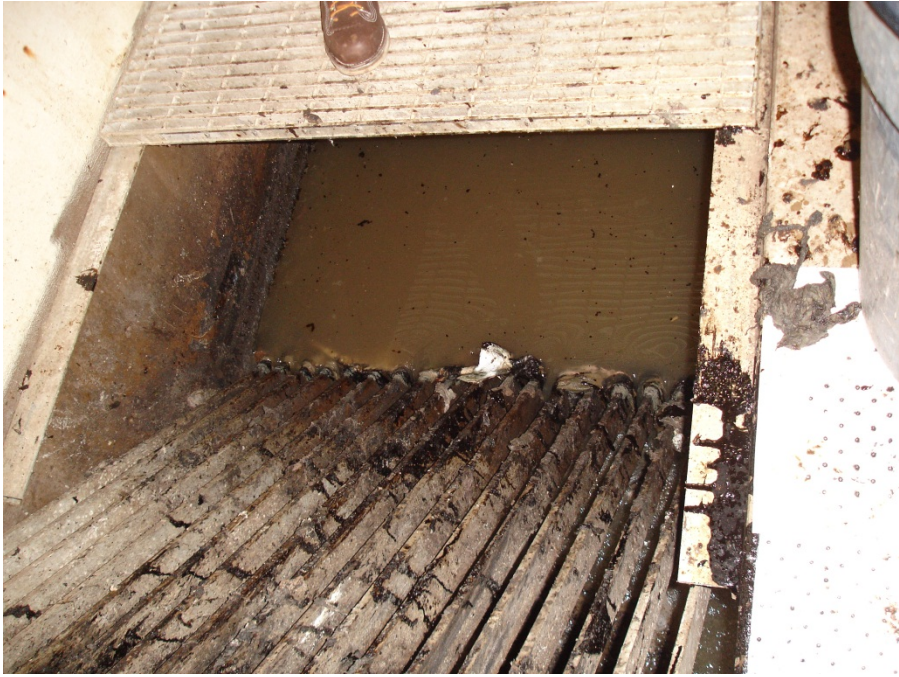
Fuel oil no. 6 contaminated equipment at WWTP pretreatment building
