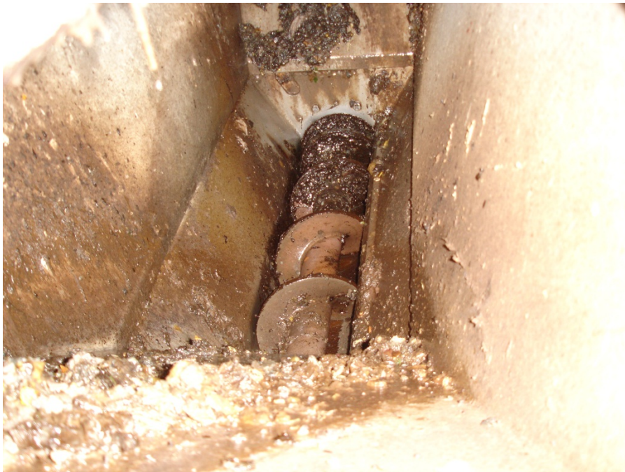
Fuel oil in waste auger at WWP pretreatment building
