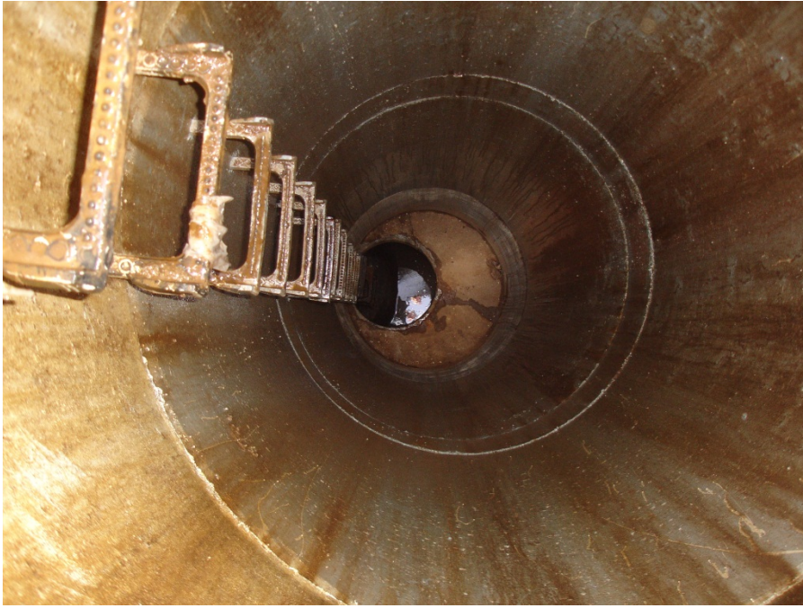
Deep manhole at WWTP
