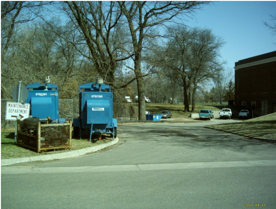
Sewage from the METO was pumped over the ground by the blue pumps shown to the left so that the half-mile of sewer could be cleaned
