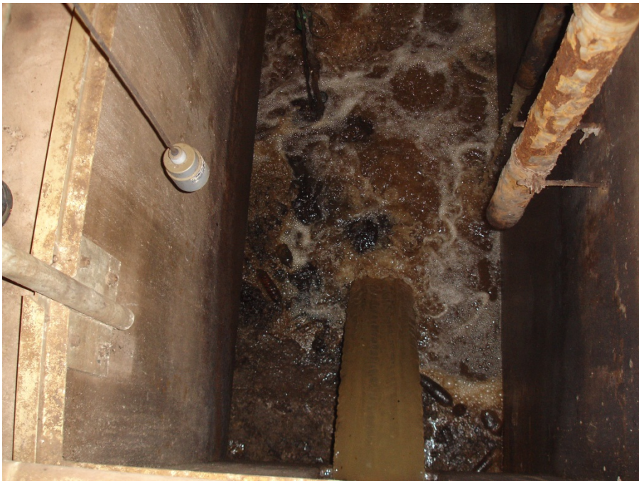
Deep pit or sump at WWTP pretreatment building contaminated with fuel oil
